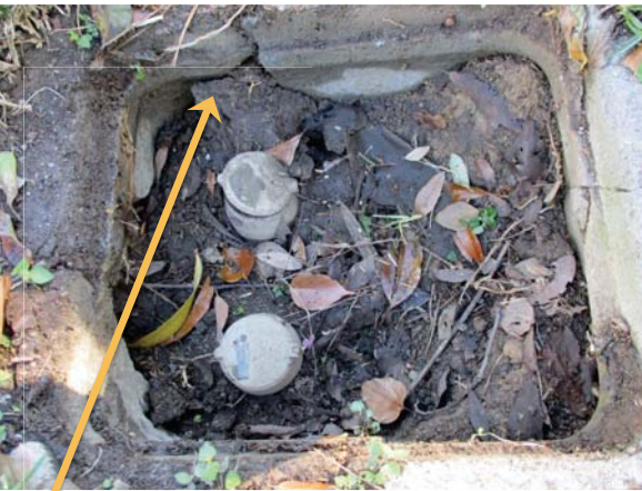
Broken Boxes and Full of Mud
