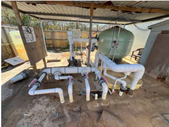
Photo #55 View of pool recirculation piping penetrations.
