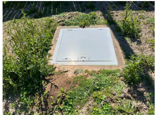
Photo #4 View of site well (lid closed) adjacent to Splashpad mechanical systems.
