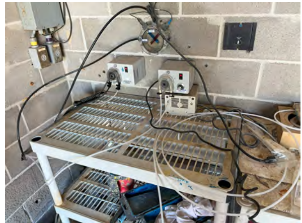
Photo #58 View of pool sodium-hypochlorite and muriatic acid chemical feed system pumps.
