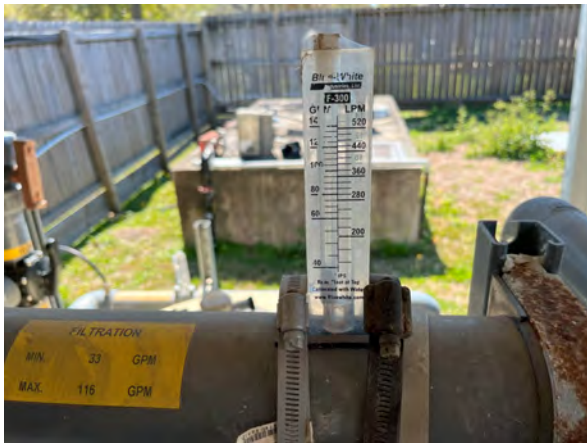
Photo #9 View of Splashpad impact flow meter.
