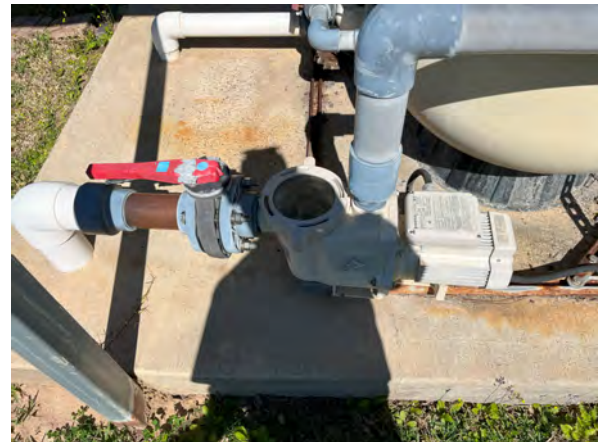
Photo #16 View of Splashpad recirculation/feature pump.
