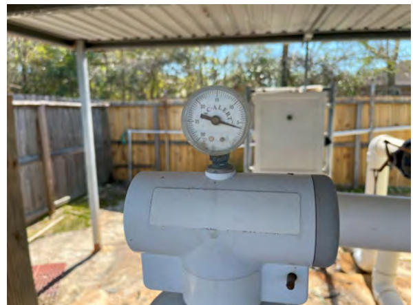
Photo #54 View of pool main drain safety vacuum release system (SVRS) pressure gauge.
