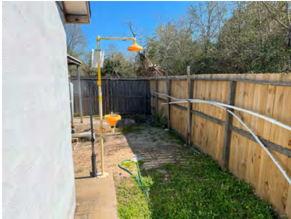
Photo #43 View of electrical conduit along south fence of mechanical area and nonoperational emergency eyewash shower.
