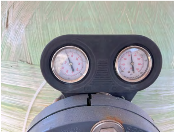
Photo #49 View of pool filter pressure gauges.
