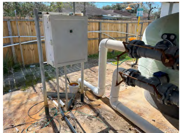
Photo #48 View of pool recirculation pump motor starter (lid closed).
