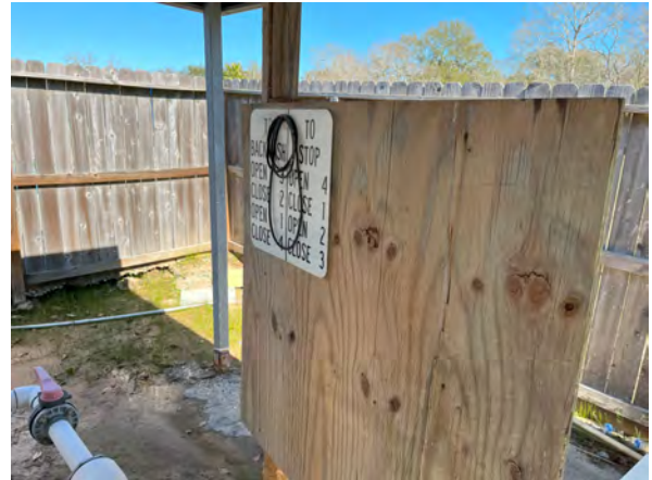
Photo #50 View of pool filter backwash sequencing directions.
