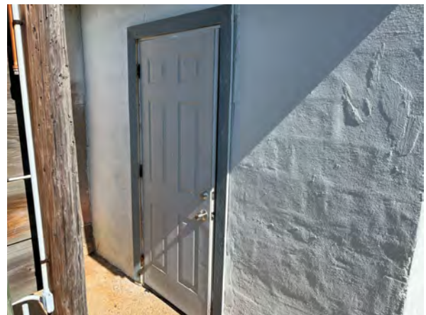
Photo #60 View pool sodium-hypochlorite storage closet entrance.
