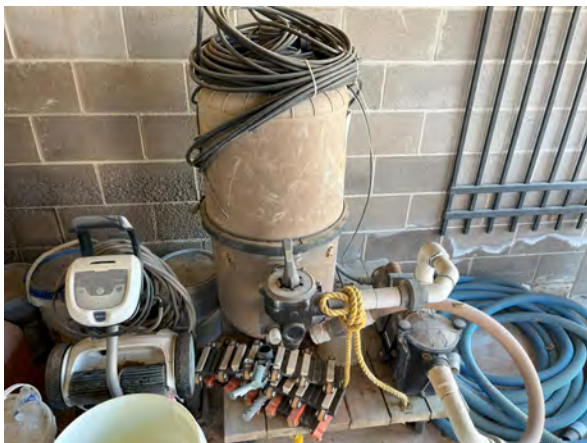
Photo #59 View of pool portable vacuum and filter system.
