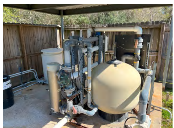
Photo #6 View of Splashpad mechanical systems.
