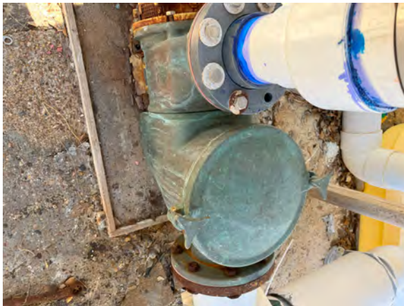
Photo #51 View of pool pump and strainer basket.
