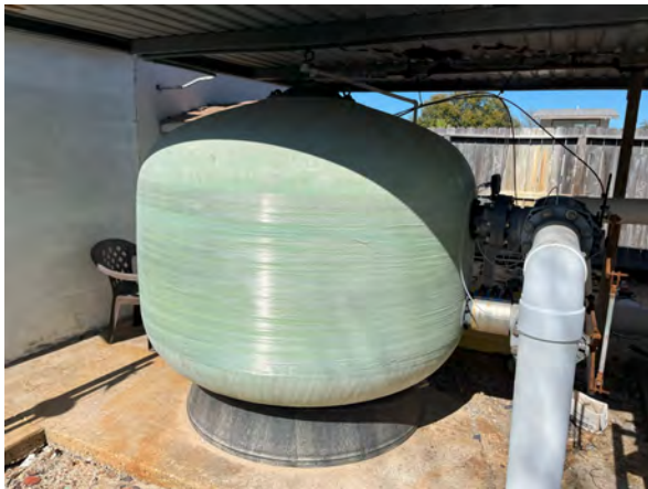
Photo #45 View of pool filter tank.
