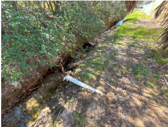
Photo #67 View of pool filter backwash line and drain down line to storm behind the pool mechanical area.
