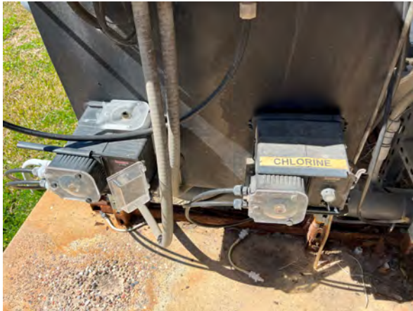
Photo #13 View Splashpad sodium-hypochlorite and muriatic acid chemical feed pumps.
