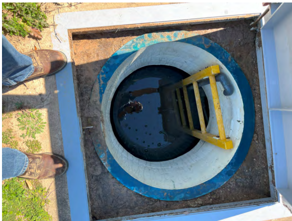
Photo #5 View of site well (lid open) adjacent to Splashpad mechanical systems.
