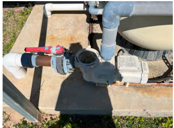
Photo #16 View of Splashpad recirculation/feature pump.
