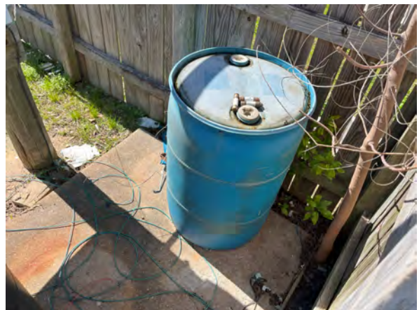
Photo #42 View of empty chemical storage carboys adjacent to pool electrical panels.
