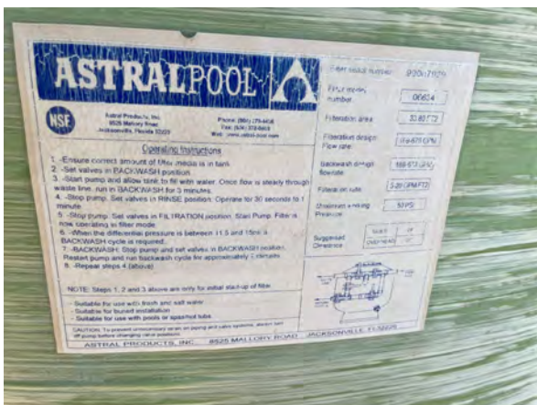
Photo #47 View of pool filter engineering specifications.
