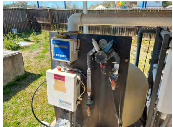
Photo #8 View of Splashpad water chemistry controller, probes, and water feature sequencing panel (lid closed).
