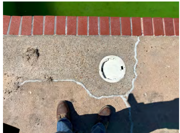
Photo #24 Example view of Children's Pool skimmer lid (cracked).
