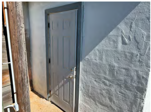
Photo #60 View pool sodium-hypochlorite storage closet entrance.
