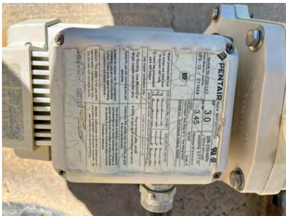
Photo #17 View of Splashpad recirculation/feature pump specifications.
