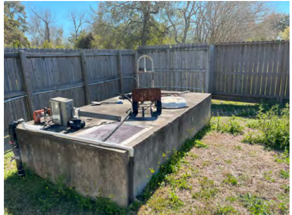
Photo #2 View of Splashpad balance tank.
