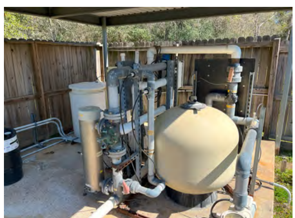
Photo #6 View of Splashpad mechanical systems.
