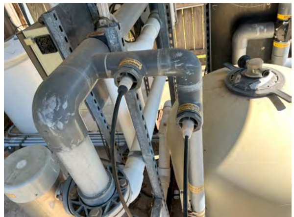
Photo #18 View of Splashpad chemical treatment system injection points.
