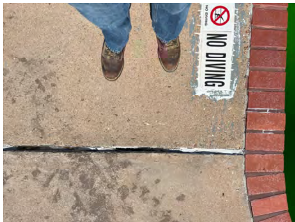
Photo #29 View of concrete deck joint with failing sealant.
