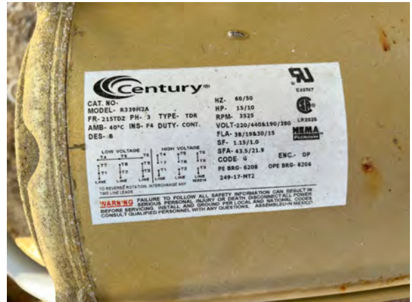
Photo #52 View of pool pump motor engineering specifications.
