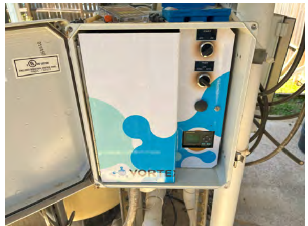
Photo #12 View of Splashpad water feature control panel (lid open).
