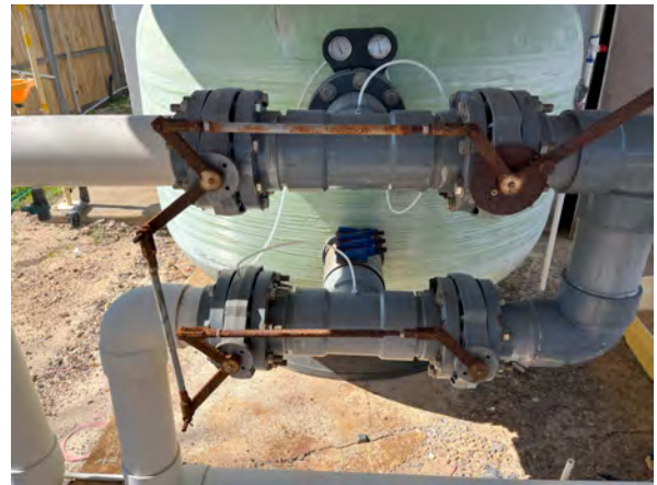
Photo #46 View pool filter face piping and valves.
