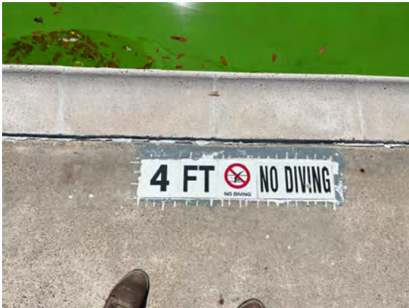
Photo #33 Example view of Lap Pool depth marking and "No Diving" signage.
