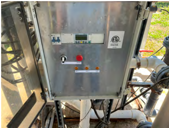
Photo #15 View Splashpad secondary disinfectant UV system control panel (lid open).
