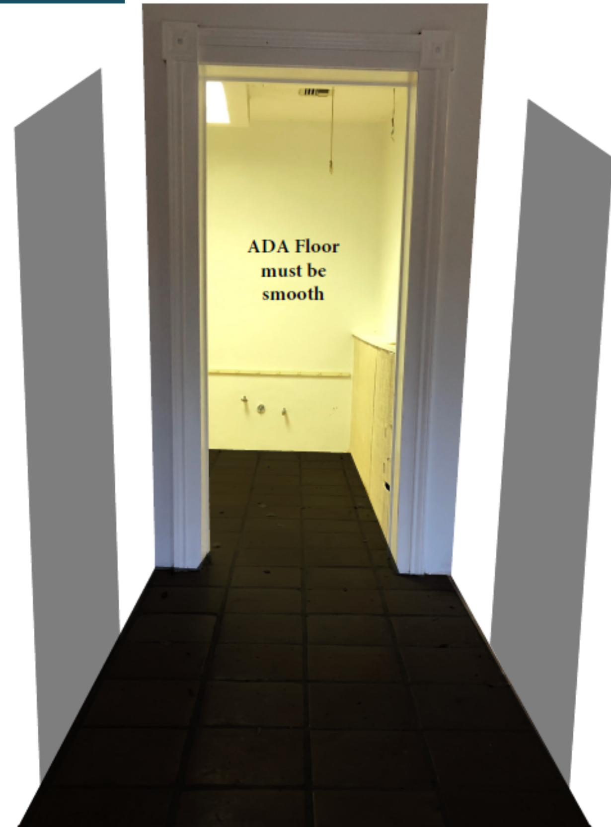
Flooring would have to be modified for ADA
