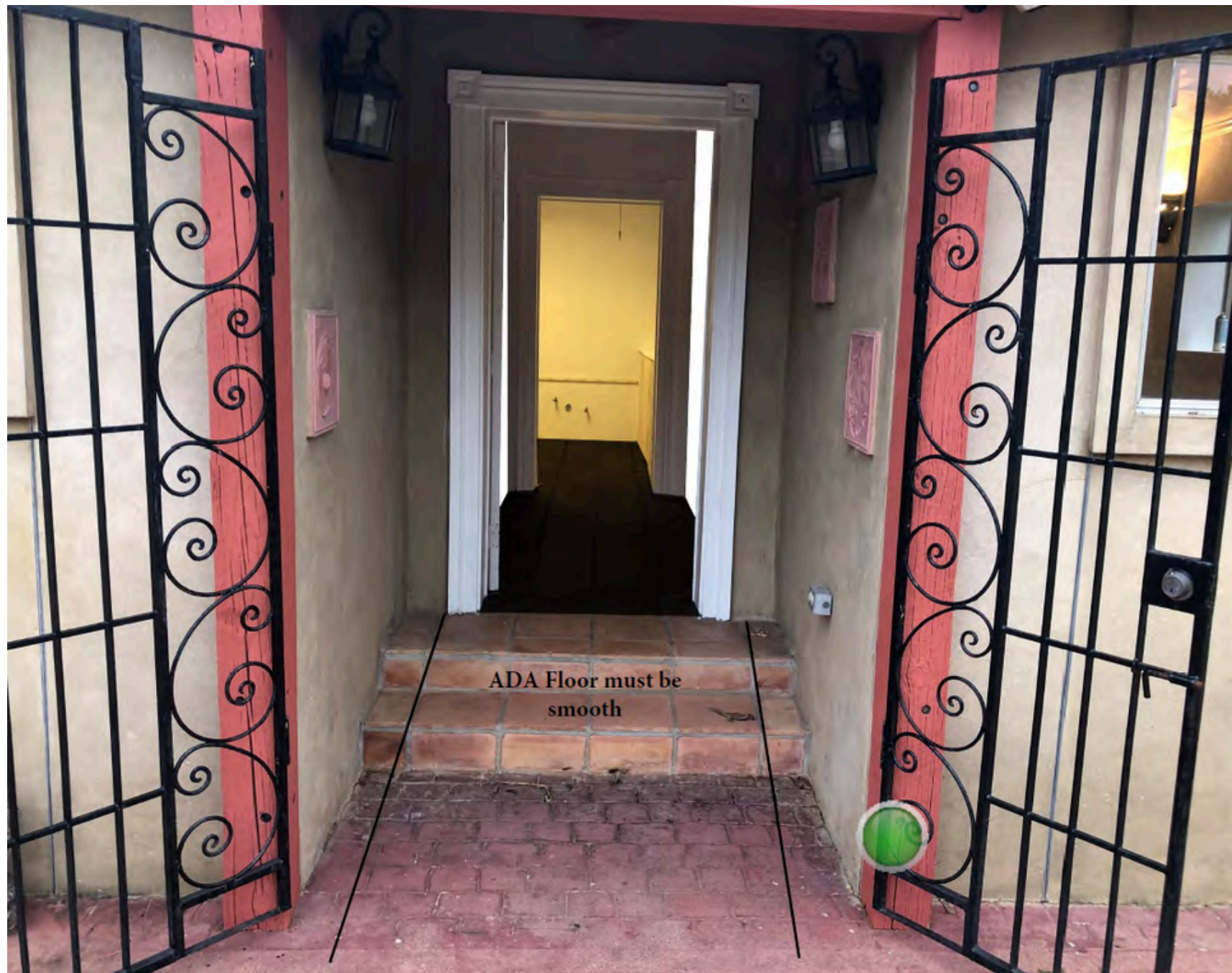
Entrance will have to have an ADA ramp
