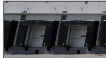
#3 INSULATED OVERHEAD DOORS WITH DOCK SHELTERS
