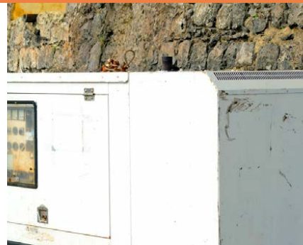
FAC 24 Generator Community Hse
