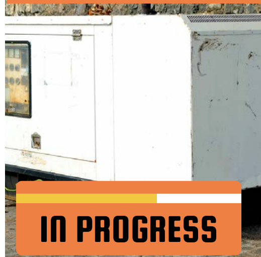
FAC33 Generator Fire Station
