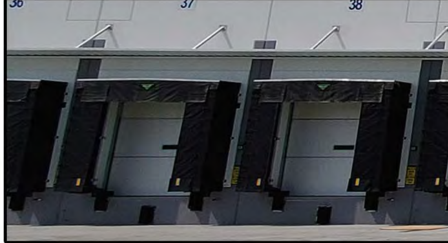
#3 INSULATED OVERHEAD DOORS WITH DOCK SHELTERS
