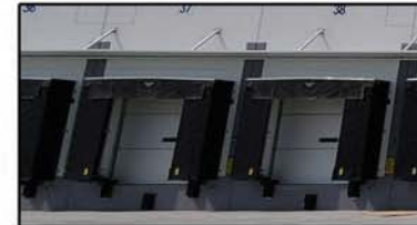
#3 INSULATED OVERHEAD DOORS WITH DOCK SHELTERS
