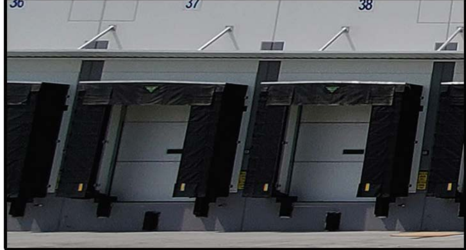
#3 INSULATED OVERHEAD DOORS WITH DOCK SHELTERS
