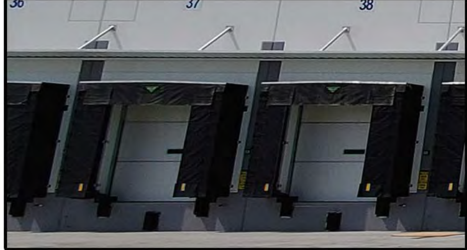
#3 INSULATED OVERHEAD DOORS WITH DOCK SHELTERS
