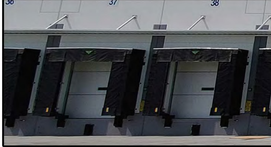
#3 INSULATED OVERHEAD DOORS WITH DOCK SHELTERS
